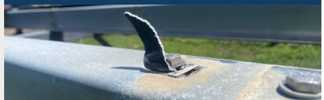
Solar module frame hole tear out, Mayreau, July 2024. Photo courtesy Chris Needham, AAS
