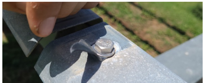
Solar module frame hole tear out. Photo courtesy Chris Needham, AAS
