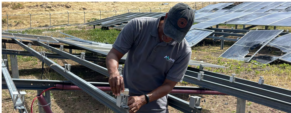
Fidel Neverson, RMI, investigating failed T-slot risers and top-down clamps on Carriacou, Grenada. Photo courtesy Skylar Bee, RMI
