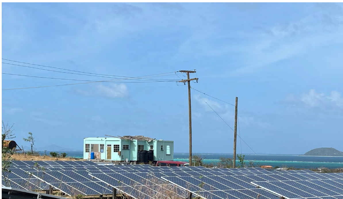
The island of Carriacou suffered through Category 5 winds from Hurricane Beryl in July 2024, but this solar array survived. Photo courtesy Christopher Burgess, RMI
