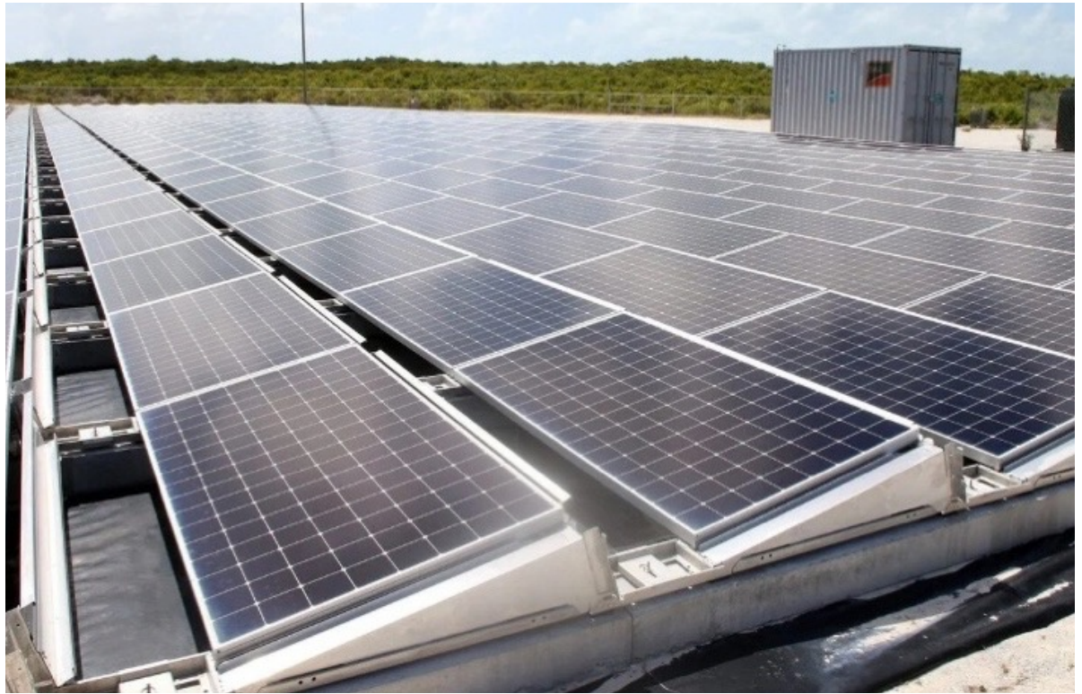
SunPower Helix mounting on Ragged Island Bahamas installed after Hurricane Irma, 2019. Photo courtesy David Kaul, Salt Energy
