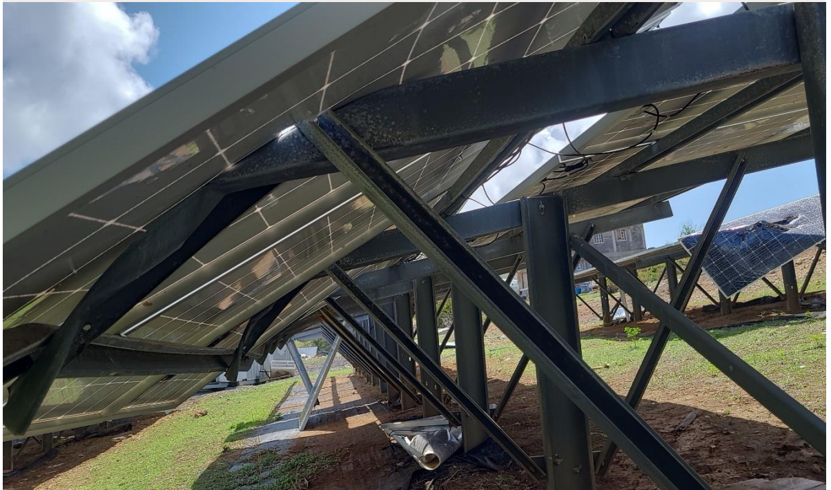
Failed solar array racking on Union Island, July 2024. Photo courtesy Frank Oudheusden, AAS
