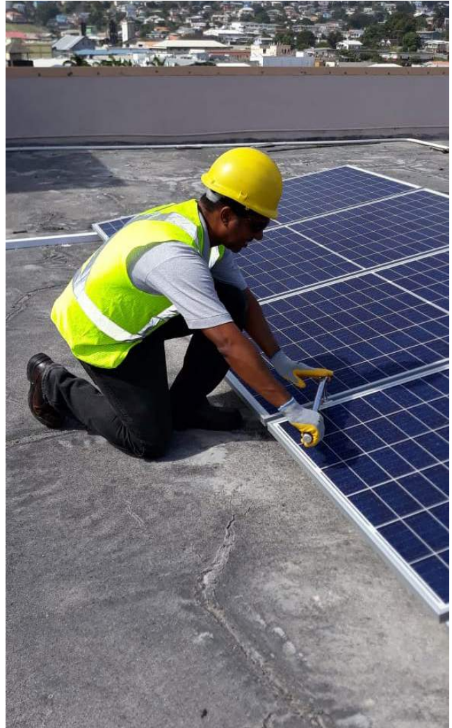
Image courtesy of Fidel Neverson, Energy Solutions, Inc.
