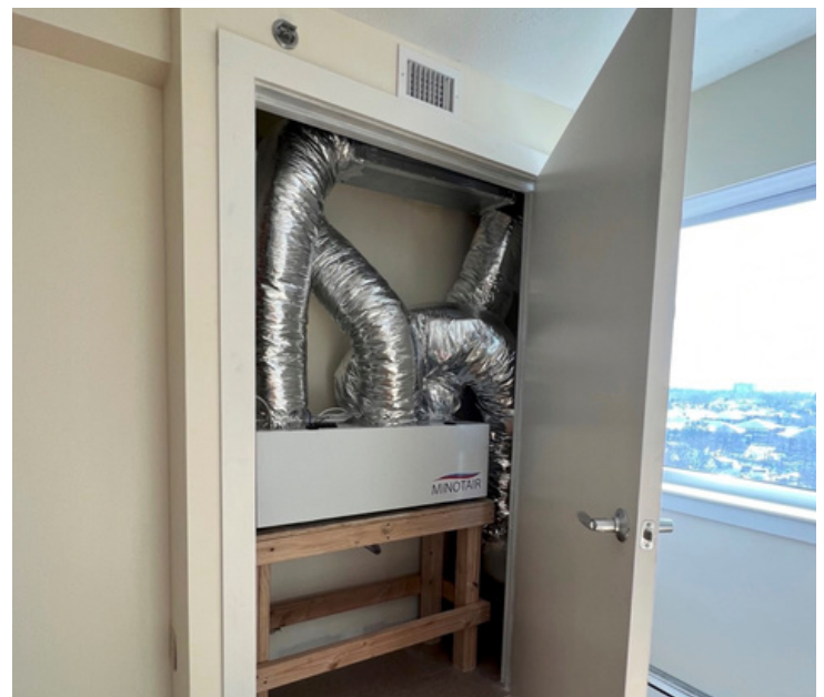
A Minotair heat pump and heat exchanger was installed in a new mechanical closet on the outside wall of each apartment.
