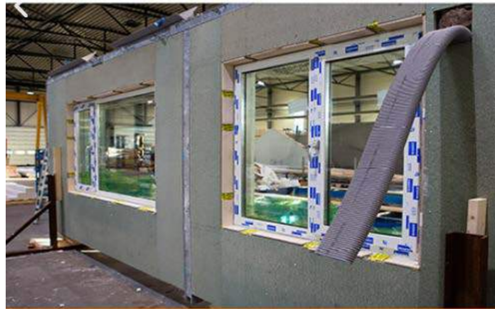
Figure 10. Ducting integrated into Renolution facade panel
