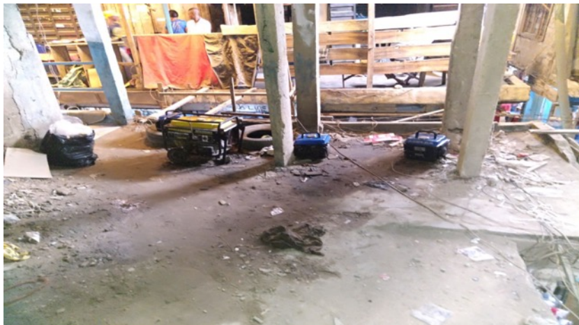
Private generators used to augment supply from the general generators
