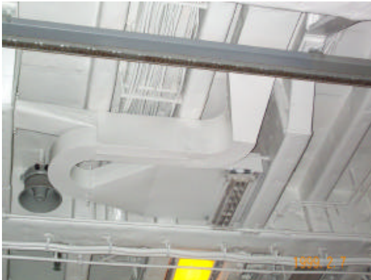
Ductwork in CG-59's hangar bay. Note the convoluted entering conditions, including a 270° bend in airflow. Jim Rogers photo.
