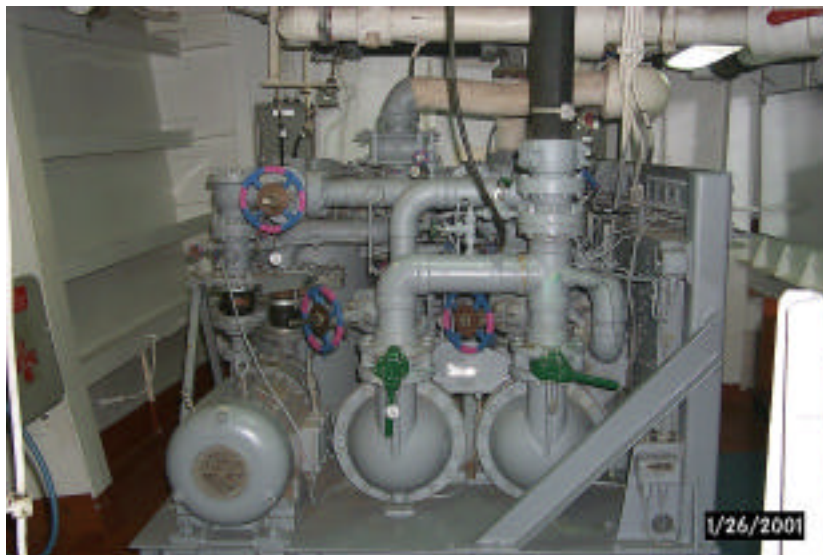
Equipment cooling heat exchanger. Ron Perkins photo.
