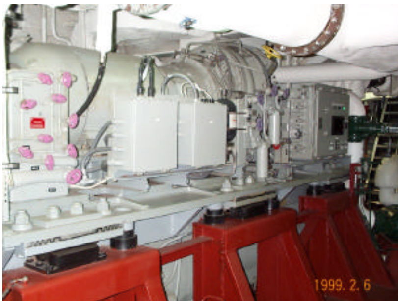
Chiller One. Ron Perkins photo (camera date was mis-set).
