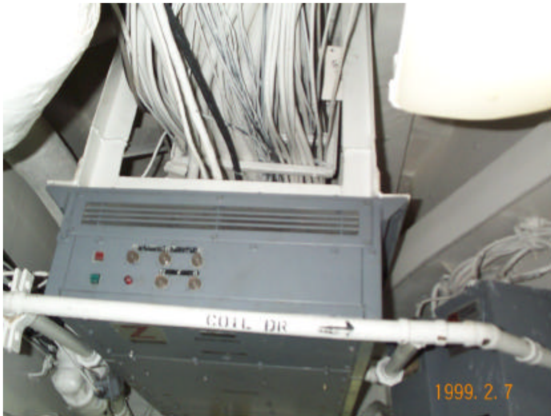
Overhead fan coil unit. Jim Rogers photo (camera date was mis-set).
