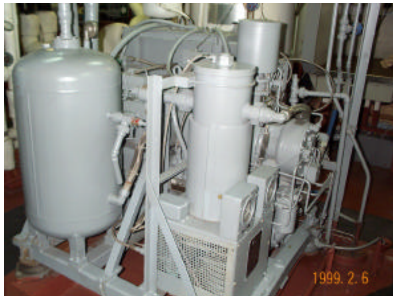
LPAC compressor skid. Jim Rogers photo (camera date was mis-set).
