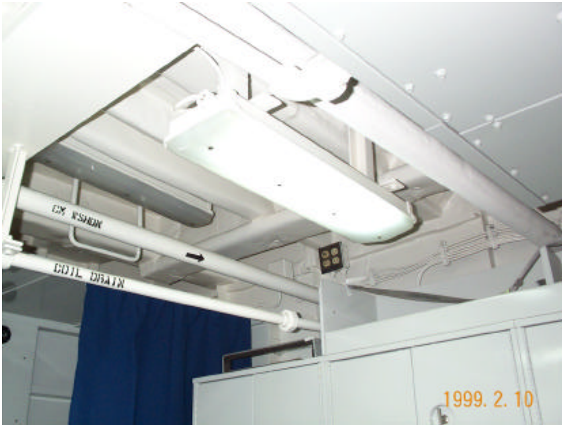
Typical overhead lighting fixture. Jim Rogers photo (camera date was mis-set).
