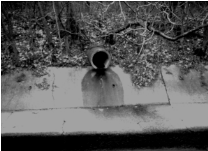
A storm sewer outfall along the channelized portion of Nine Mile Run.
