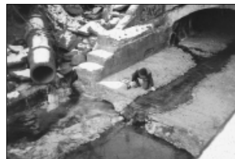
The outfall of the main Nine Mile Run culvert at low flow...
