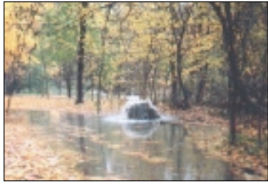
Surcharged with stormwater, a manhole structure on a sewer line in Frick Park overflows, spilling contaminated water into the park. Photograph by Mike Lichte, Allegheny County Health Department.
