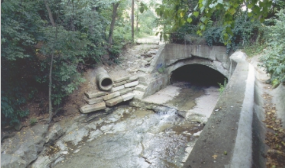
Existing conditions at the Nine Mile Run culvert outfall. Photograph by Richard Pinkham, RMI.
