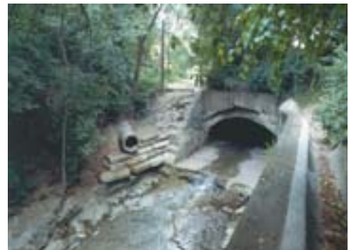
Before and after: Photo of a Pittsburgh culvert outfall today (this page) and a drawing of how the culvert would appear if creatively designed (next page)
