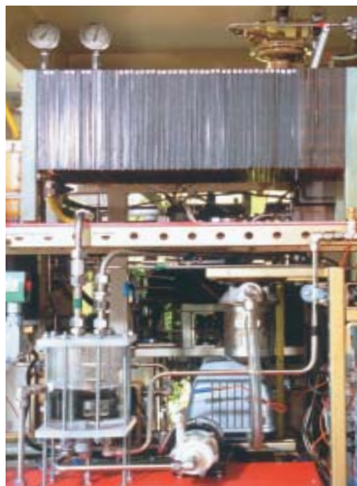
This 1.0 kW proton exchange membrane (PEM) fuel cell uses solar hydrogen to run the Telonicher Marine Lab air compressor in Trinidad, California when the sun is not shining. Electricity from photovoltaic panels runs the air compressor when the sun is shining.
