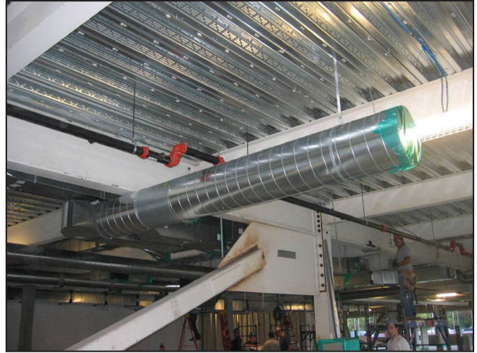
Figure 4: The later addition of ductwork revealed the intelligence of BIM and its users. (Since water will rarely flow in the sprinkler pipe, the orthogonal bends do not significantly increase pumping energy use.) Image courtesy of Tocci Building Corporation.
