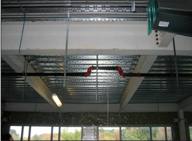
Figure 3: The sprinkler pipe was assembled before the ductwork, showing off a surprising bend. Image courtesy of Tocci Building Corporation.
