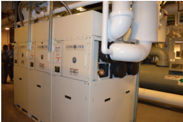
The CCB's new geothermal heat recovery chiller.
