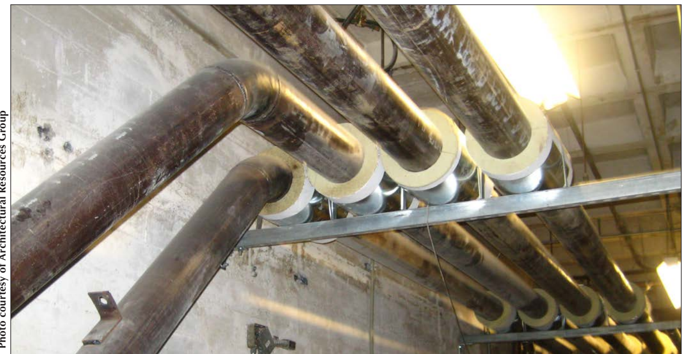
Piping design with gradual bends in Caltech's Linde + Robinson Laboratory building is more efficient than piping design with 90 degree angles because it reduces friction losses along the length of the pipe.
