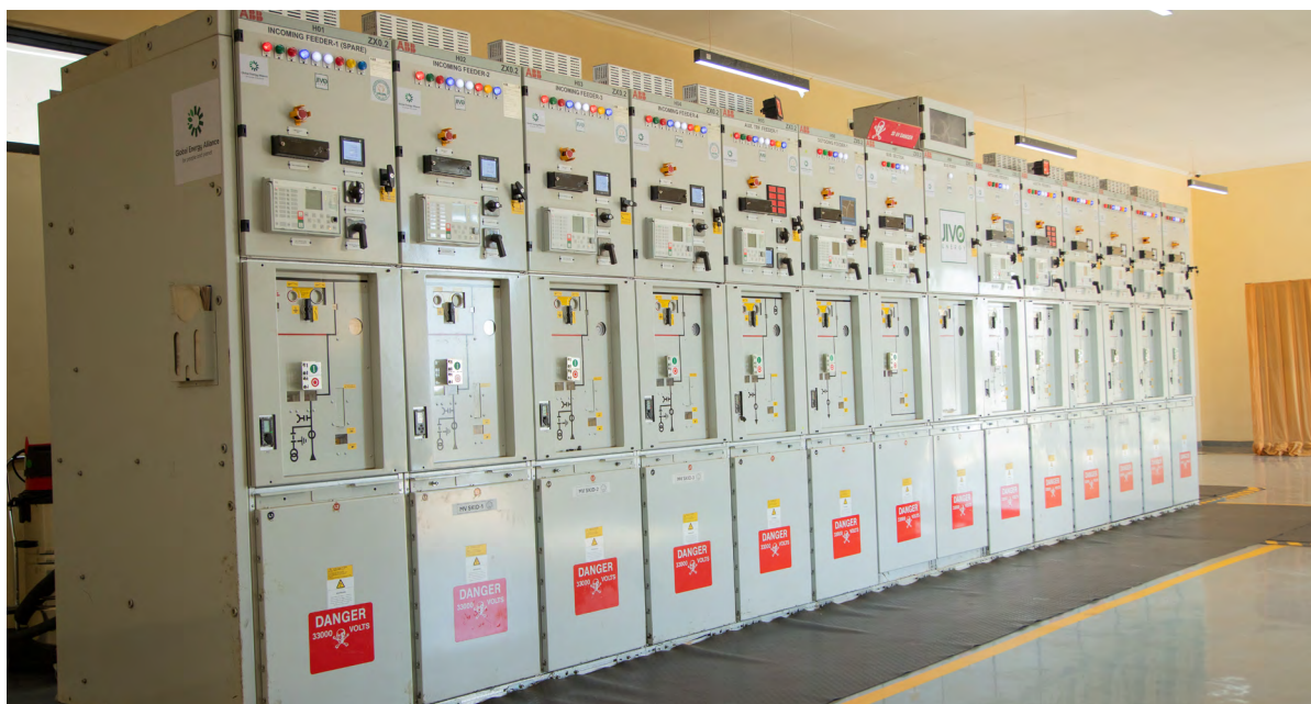
Gas-insulated switchgear at the BESS facility in Kanengo, Lilongwe, Malawi.
