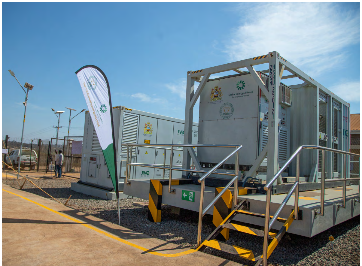
BESS facility at Kanengo, Lilongwe, Malawi.
