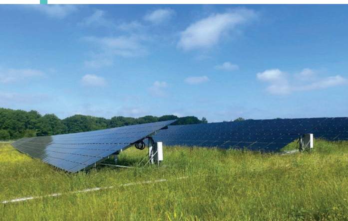
This 4 megawatts solar project, in Cuyahoga County, Ohio, supplies enough electricity to power 500 homes. Photo courtesy of Jackie Lombardi
